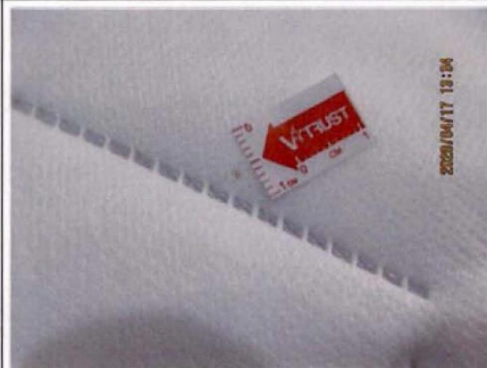
† 22 - Slight dirt stains on unit - minor
